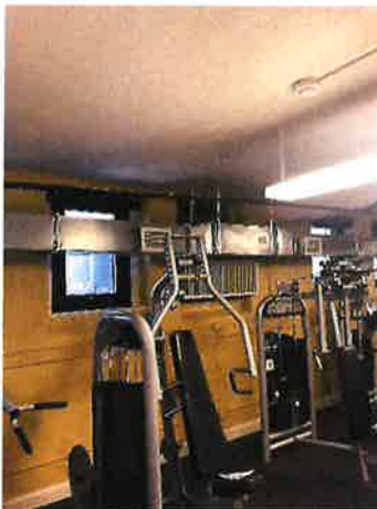
Fitness Center Ductwork
