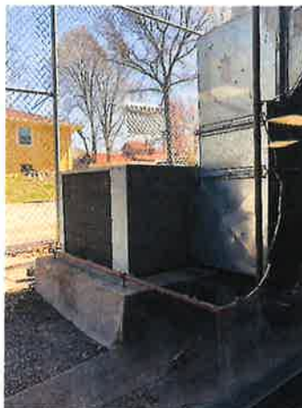
Typical Ground-Mounted RTU
