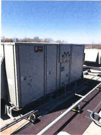
Typical Gymnasium 15-Ton RTU
