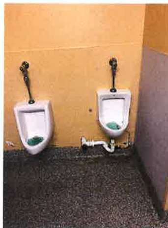
Urinals with Water Damage
