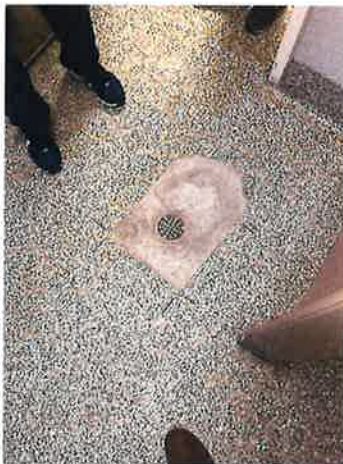
Patched Floor Drain
