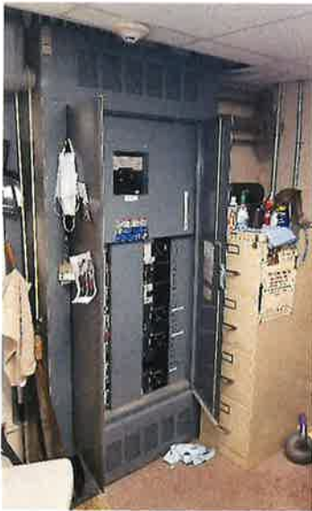
Main Service Panel MDP
