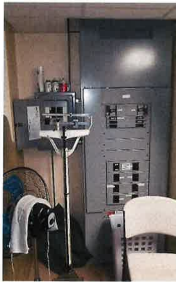
Panelboard DP1 adjacent to MDP
